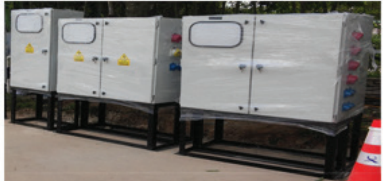
DB PANEL & TRANSFORMER
